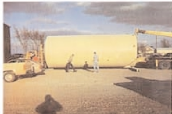
12' x 34' Vertical Tank with 2" Insulation and Heat Tracing
